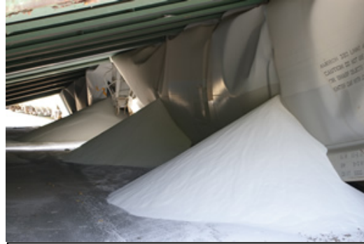
Minneapolis I-35W collapsed bridge damage.
